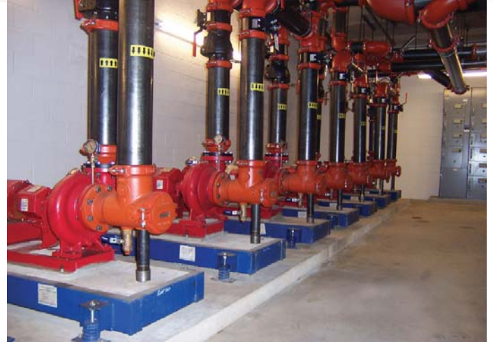
The HVAC water circulation pumps.
