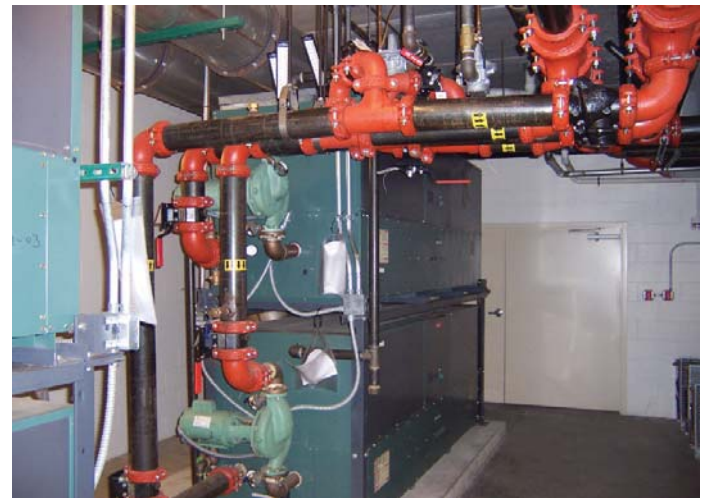
The gas-fired boilers for winter heating.
